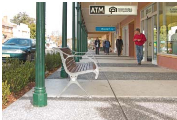
Footpath, street furniture and landscaping works in Bridge Street Muswellbrook completed in 2016.
