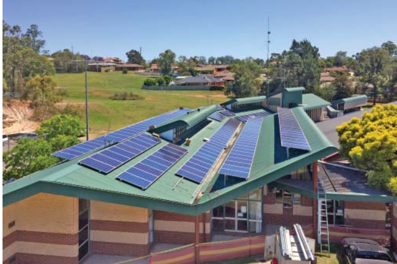
In 2016 Council buildings were fitted with a total of 237kw of solar panels.
