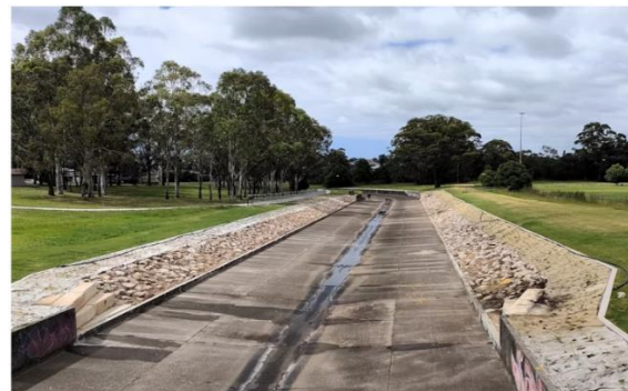
We replaced 300m of concrete channel wall with sandstone rocks along the embankment to create a more natural environment.
