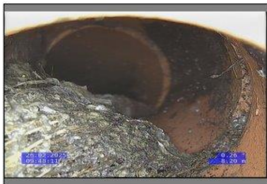
Photo: 357_358_2292_A.JPG 8.2m. Defective junction, roots are growing into and/or down the connecting conduit, magnitude of obstruction 5-20% , at 9 o'clock
