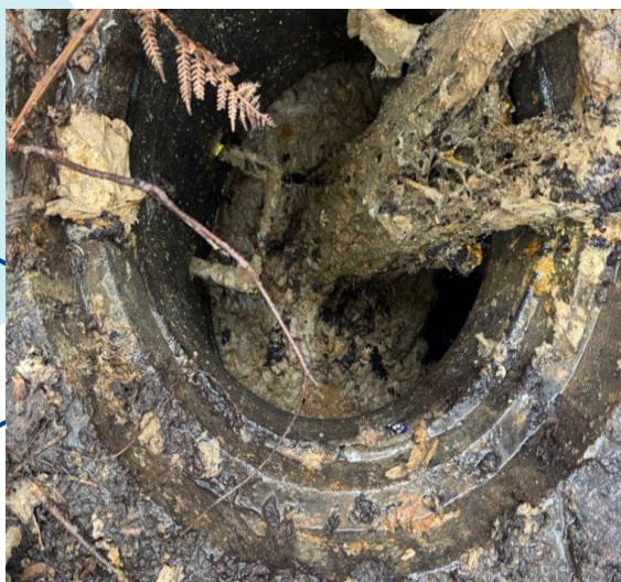
A "fat berg" at a sewerage manhole
