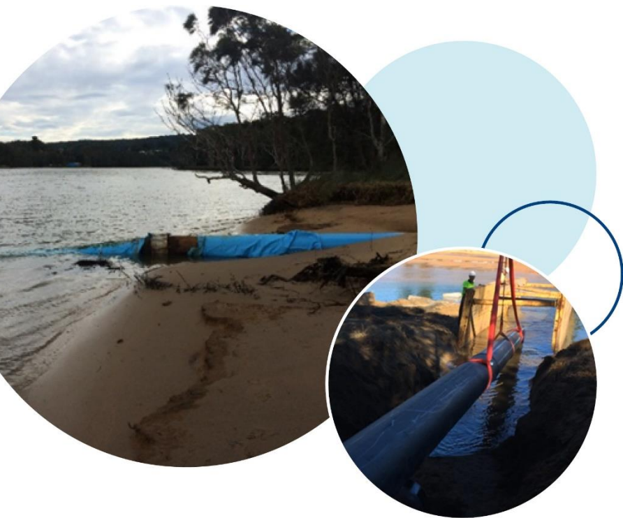
Previous repairs undertaken to original 450mm diameter cast iron cement lined trunk main
