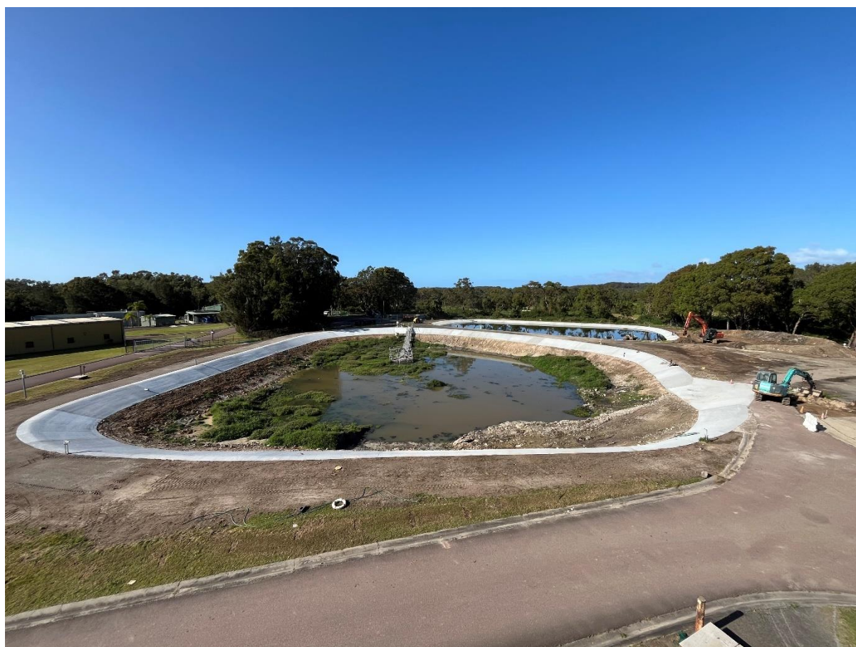
Figure 31: Toukley STP sludge lagoon
