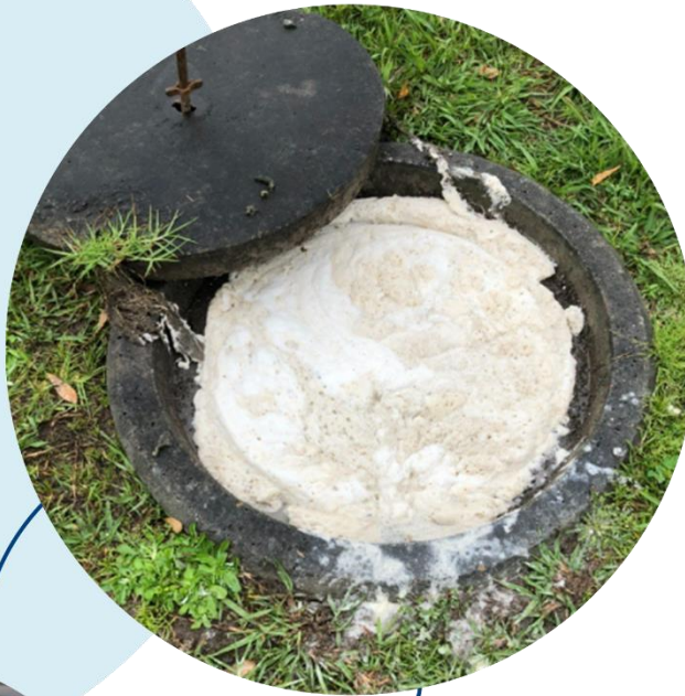
An example of fats and grease in the sewerage network
