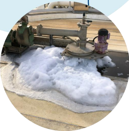
Poor quality trade waste at sewage treatment plant inlet works
