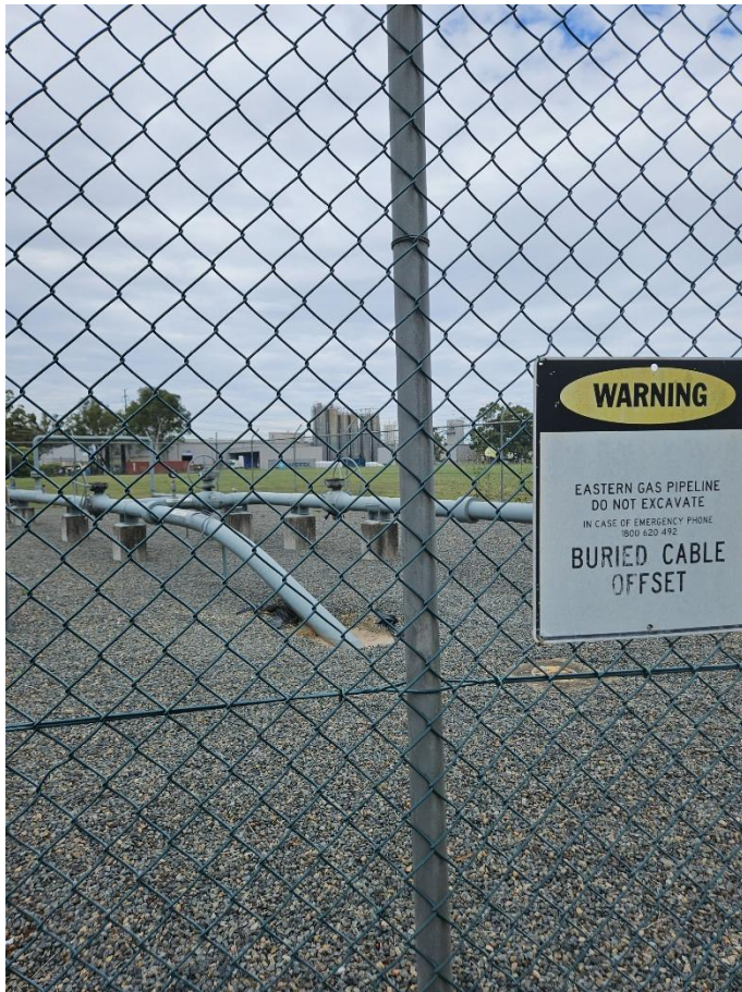
Photo Description: Natural gas pipeline
