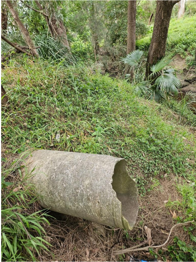
Photo Description: Derelict PACM stormwater outlet
