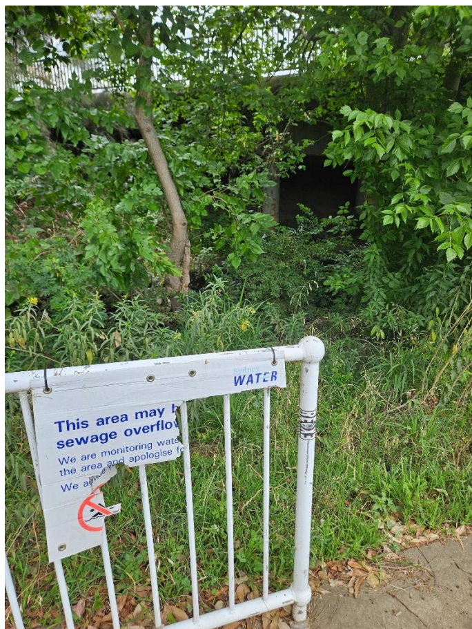
Photo Description: Sewage overflow contributes to the creek
