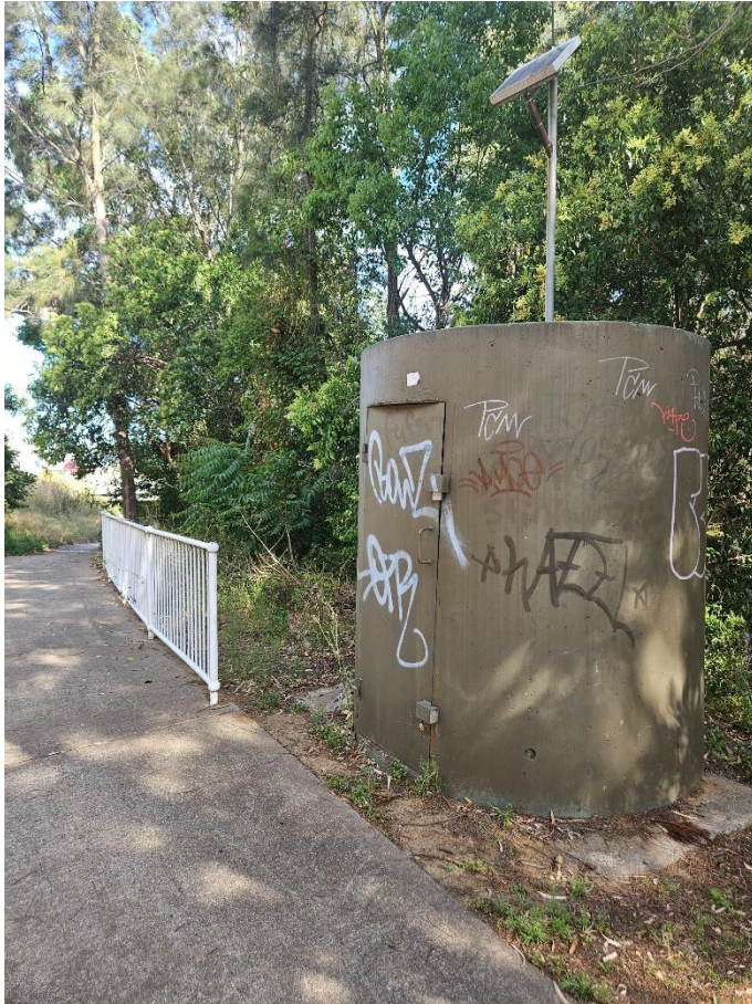
Photo Description: Above ground storage tank with solar battery adjacent the creek
