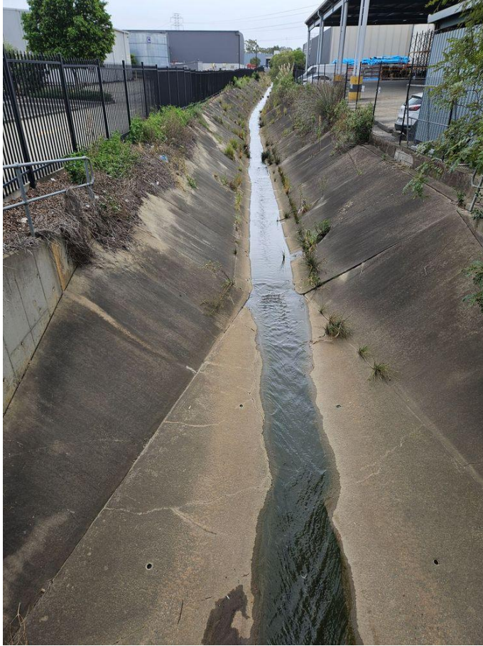
Photo Description: Facing west minimal contribution from weepage pores.
