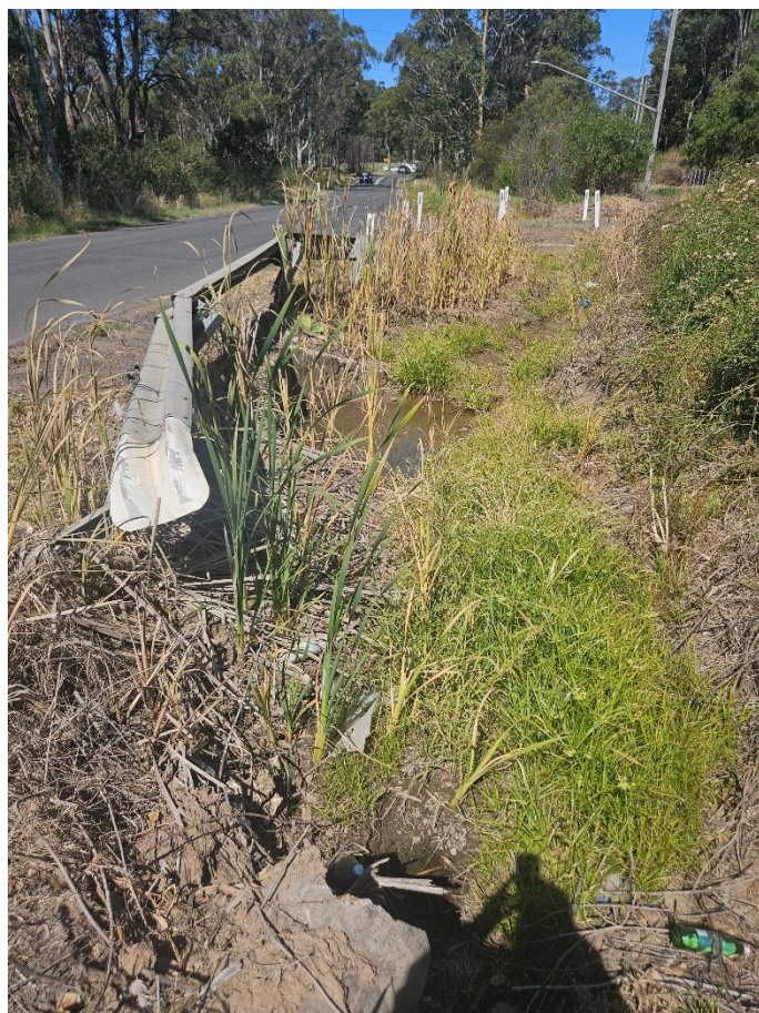
Photo Description: Sealed turnaround bay adjacent roundabout, evidence of fill.
