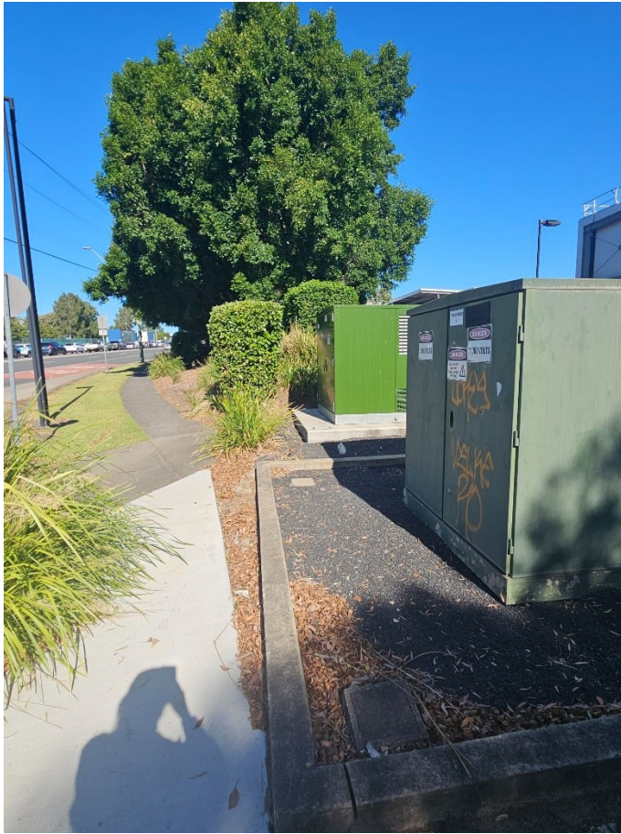
Photo Description: ASTs at BOC facility
