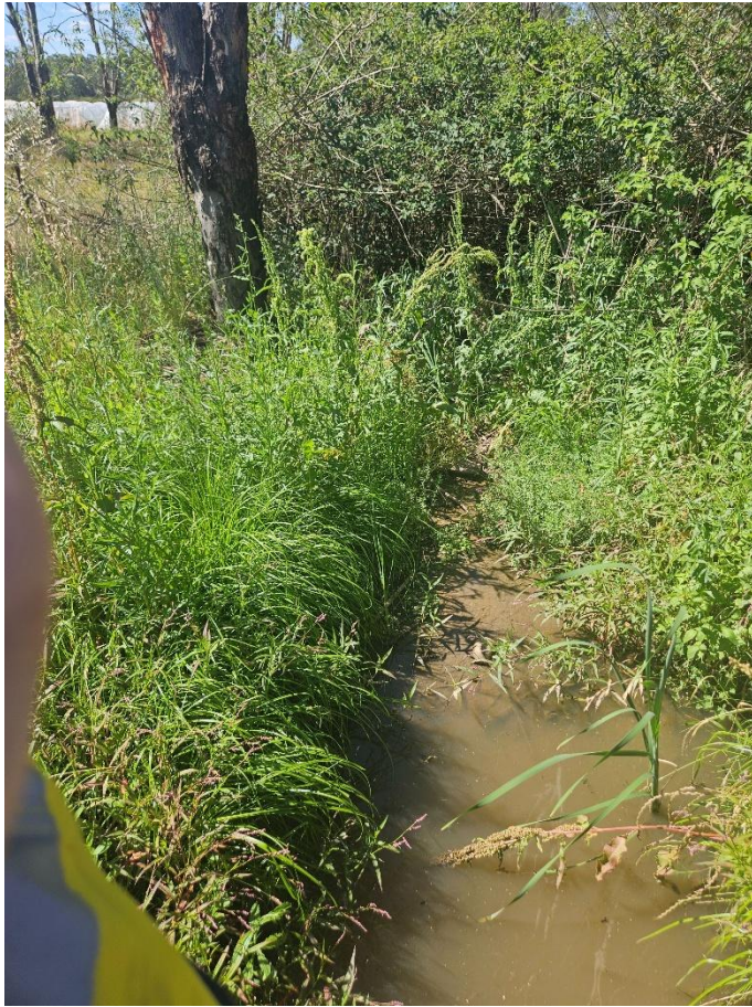
Photo Description: Offside, Stagnant drainage channel with stormwater input
