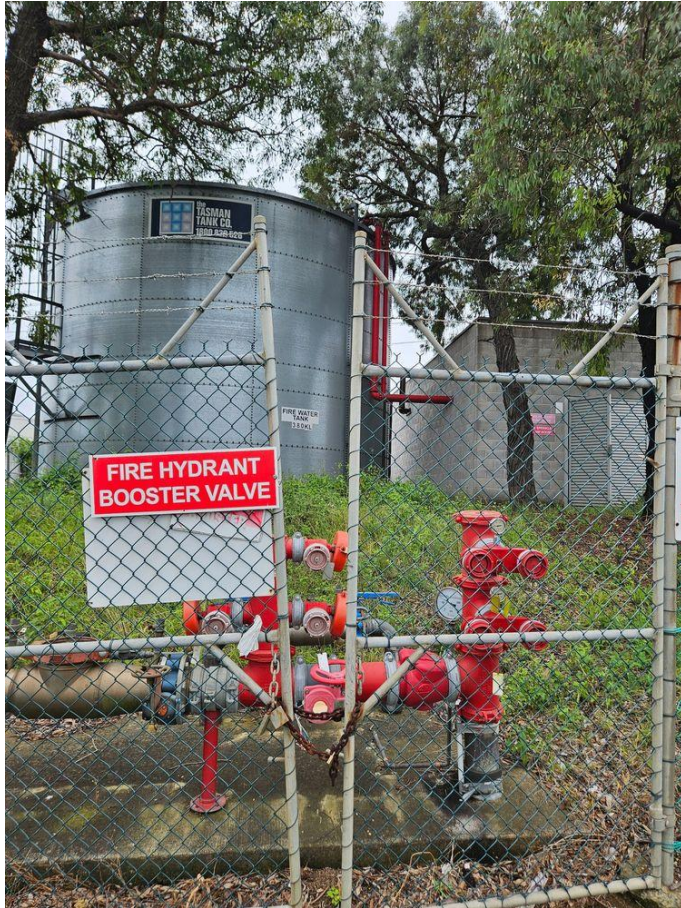
Photo Description: 380 KL fire water tank and fire pump room at Vellex
