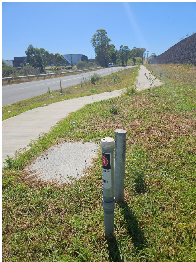
Photo Description: Jemena high pressure gas pipeline
