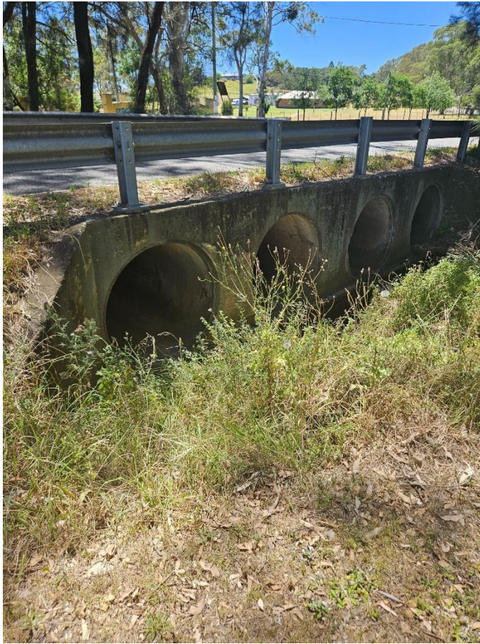
Photo Description: Reedy Ck looking south from Burley St, stagnant and discontinuous
