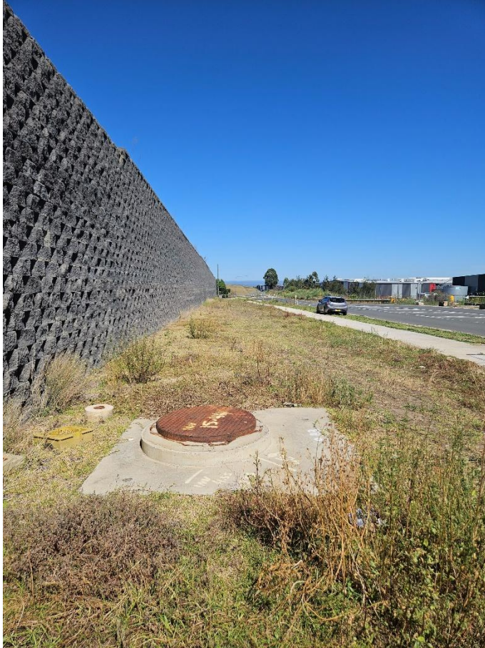
Photo Description: Sewerage infrastructure at the approximate location of the pipeline exiting the Pipeline End Lot
