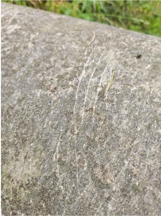
Photo Description: Derelict PACM stormwater outlet surface
