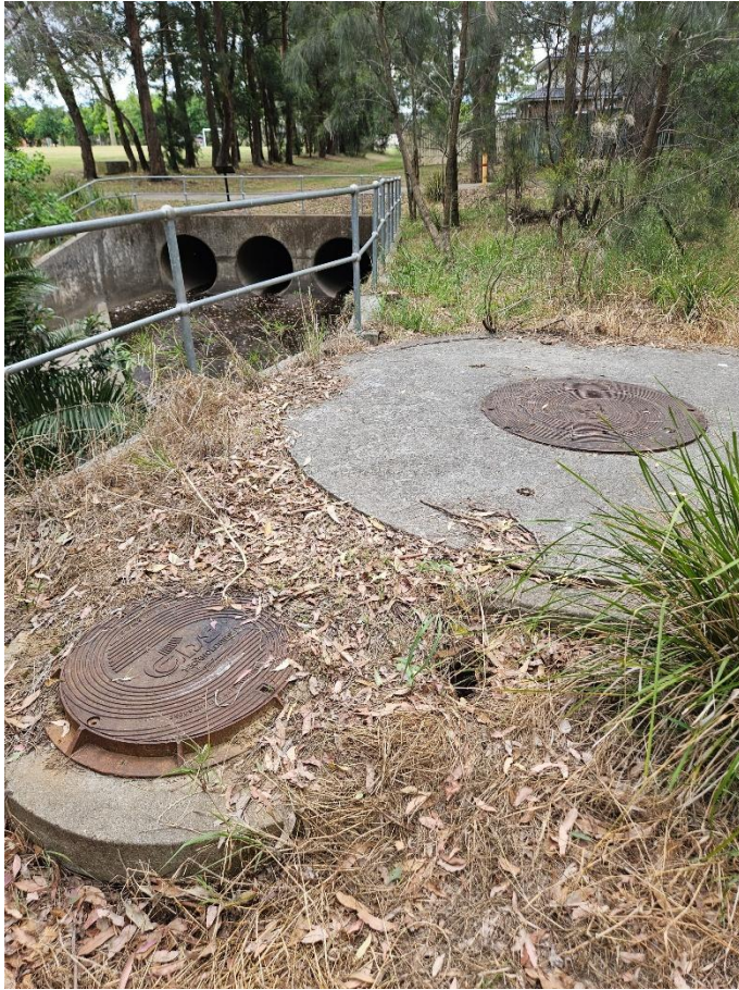
Photo Description: Stormwater USTs
