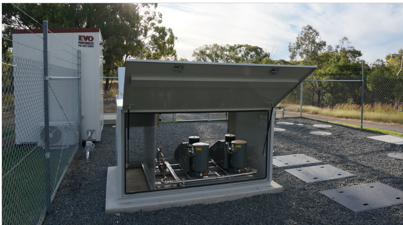
Figure 7.4 - 40kL Kubota WWTP for Water Utility - Plant room, electrical box, and monitoring unit (foreground) site office (background)
