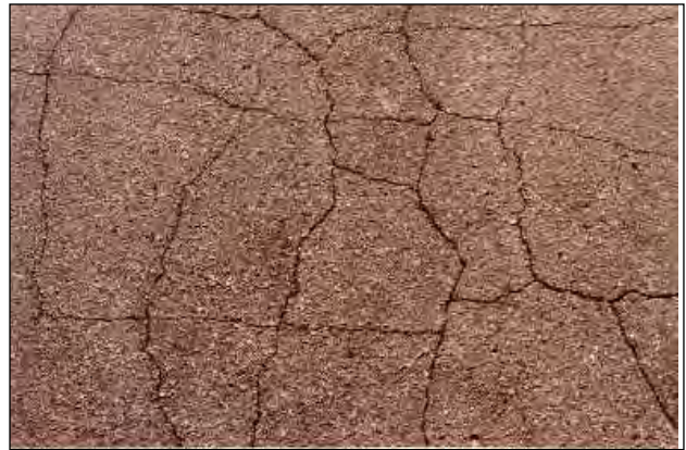
Condition 5 – Very Poor
