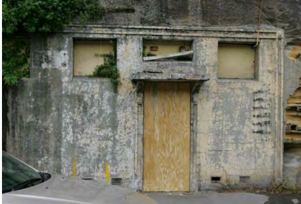
Condition 5 – Very Poor
