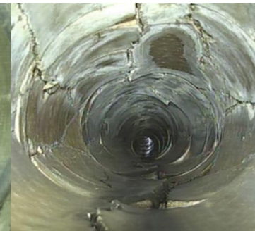
Poor/ Very poor:
