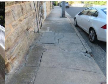
Poor/ Very poor:
