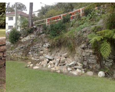
Poor/ Very poor:
