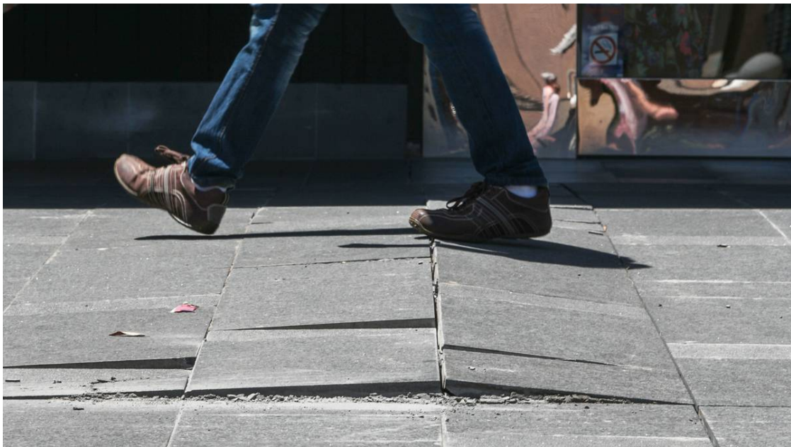
A passer-by walks over the cracks that have already appeared in the refurbished mall pavement. Picture: Adam Maclean
