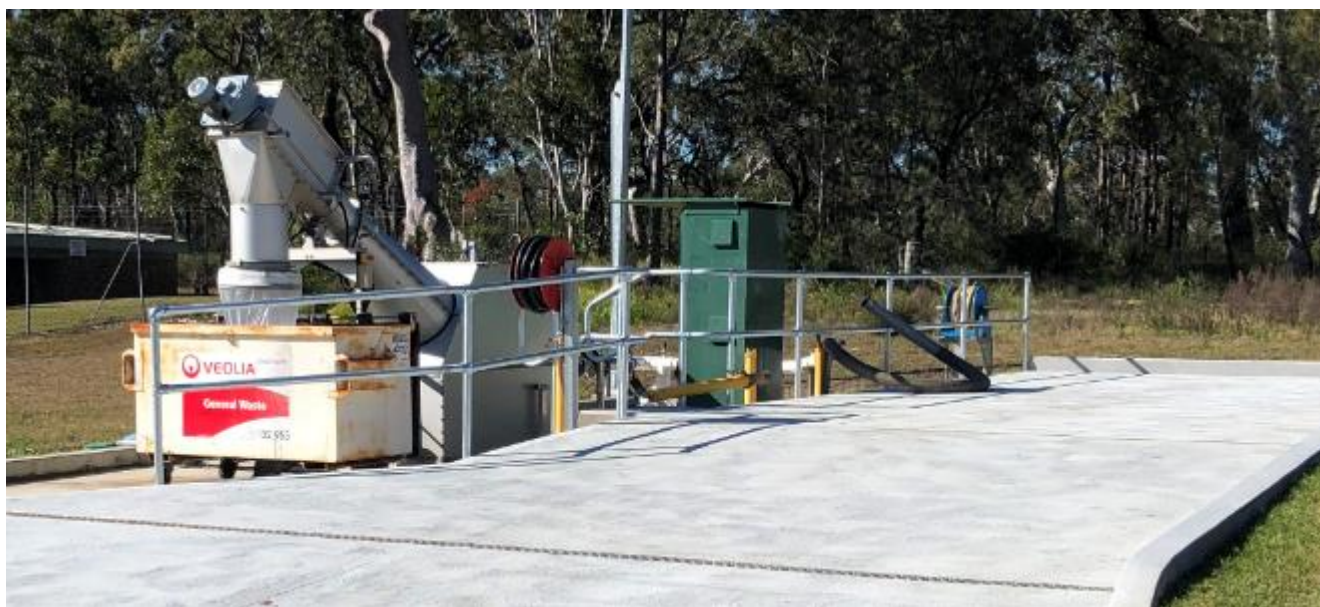
Figure 3: Septic receiving station allows for safe discharge of tankered septic waste, measurement of discharge volumes and rag removal
