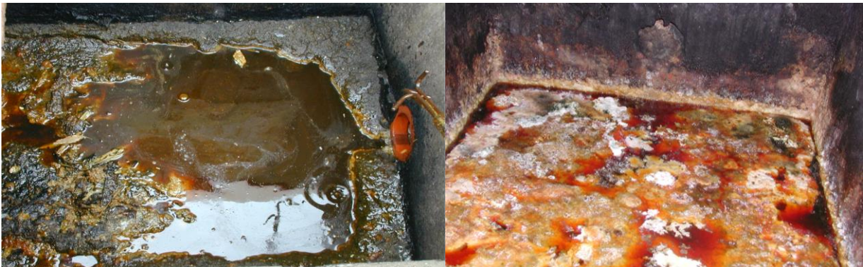
Figure 2: Poorly maintained pre-treatment devices affect downstream infrastructure
