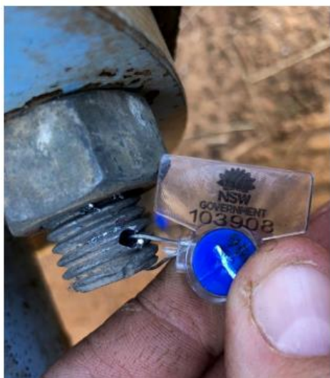
Figure 3-1 Example of an installed tamper-evident seal
