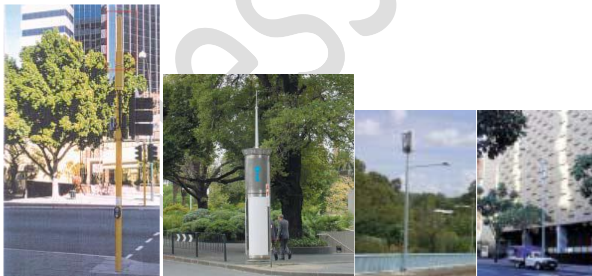
A colour matched “extension” to the traffic lights. Microcell on a CBD “smartpole”. co-location on street lights/poles.
