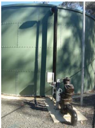
Photograph 4: Balance Tank at Pennant Hills
